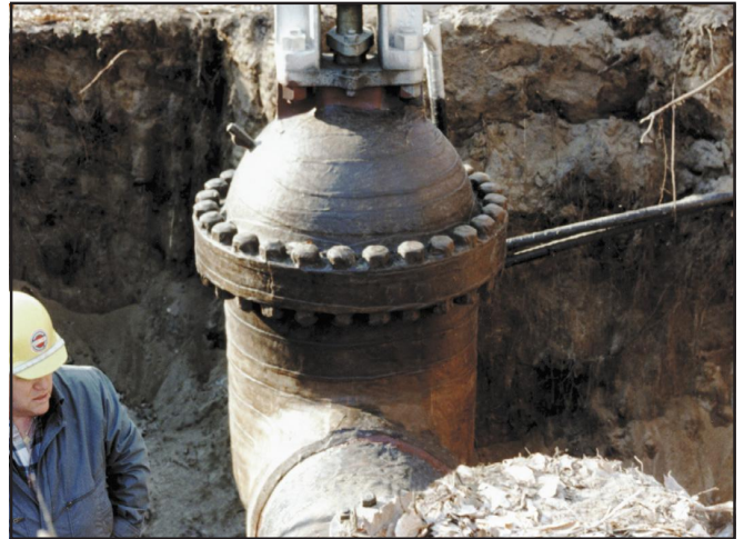
#1 Wax-tape can be applied to small and large valves, flanges and bolts
